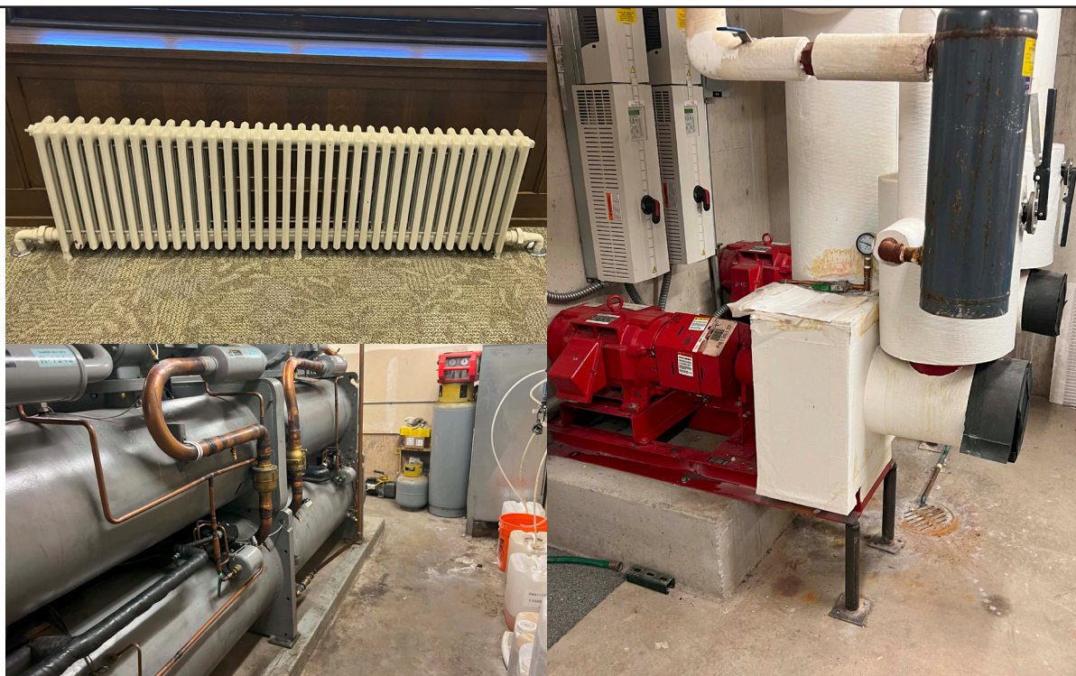
Clockwise from top left: Farnsworth Group completed field assessments for all district branches, determining facility deficiencies and recommended pathways forward for PPLD. Some of the deficiencies include HVAC air and water systems, as pictured to the right.
